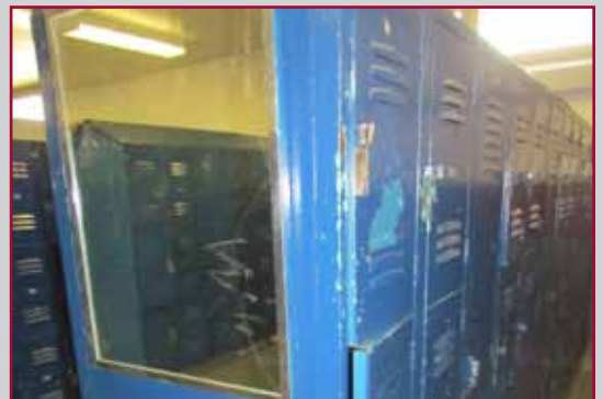
Outdated locker room to be renovated at Robert Frost.
