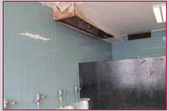
Dilapidated bathrooms to be renovated at the high school.
