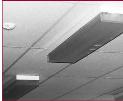
Light occupancy sensors placed in the high school classrooms will eliminate excess electrical costs.
