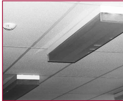
Light occupancy sensors placed in the high school classrooms will eliminate excess electrical costs.
